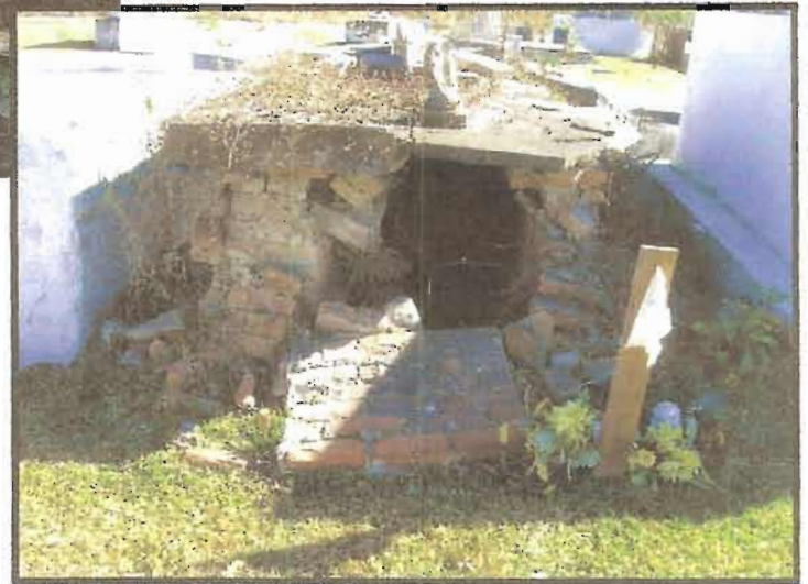
Above: Damage done to the historic brick by the application of an inappropriate stucco
