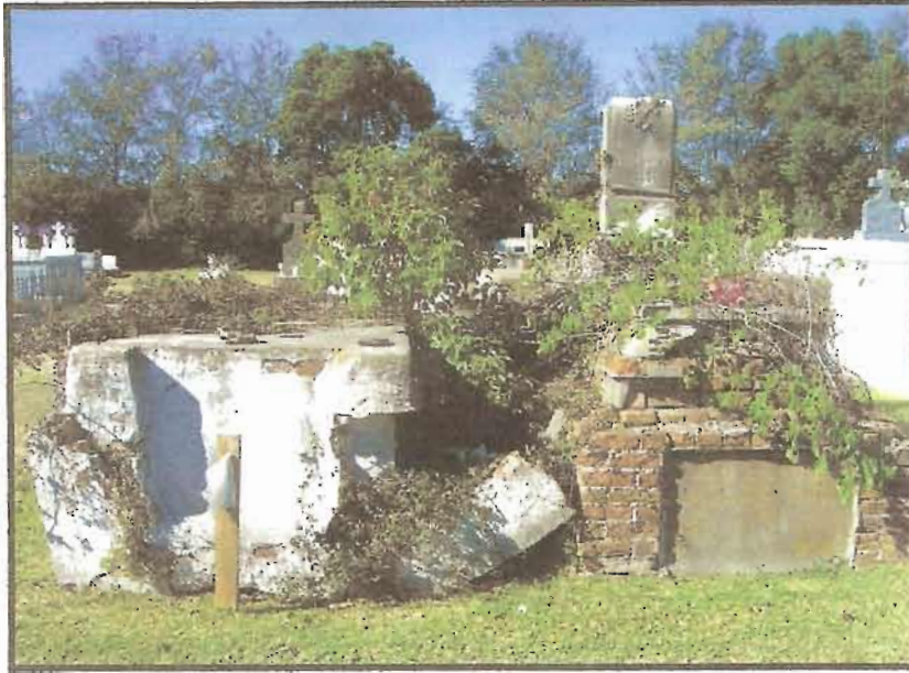
Above: Representative condition of several historic tombs in Patoutville Cemetery.
